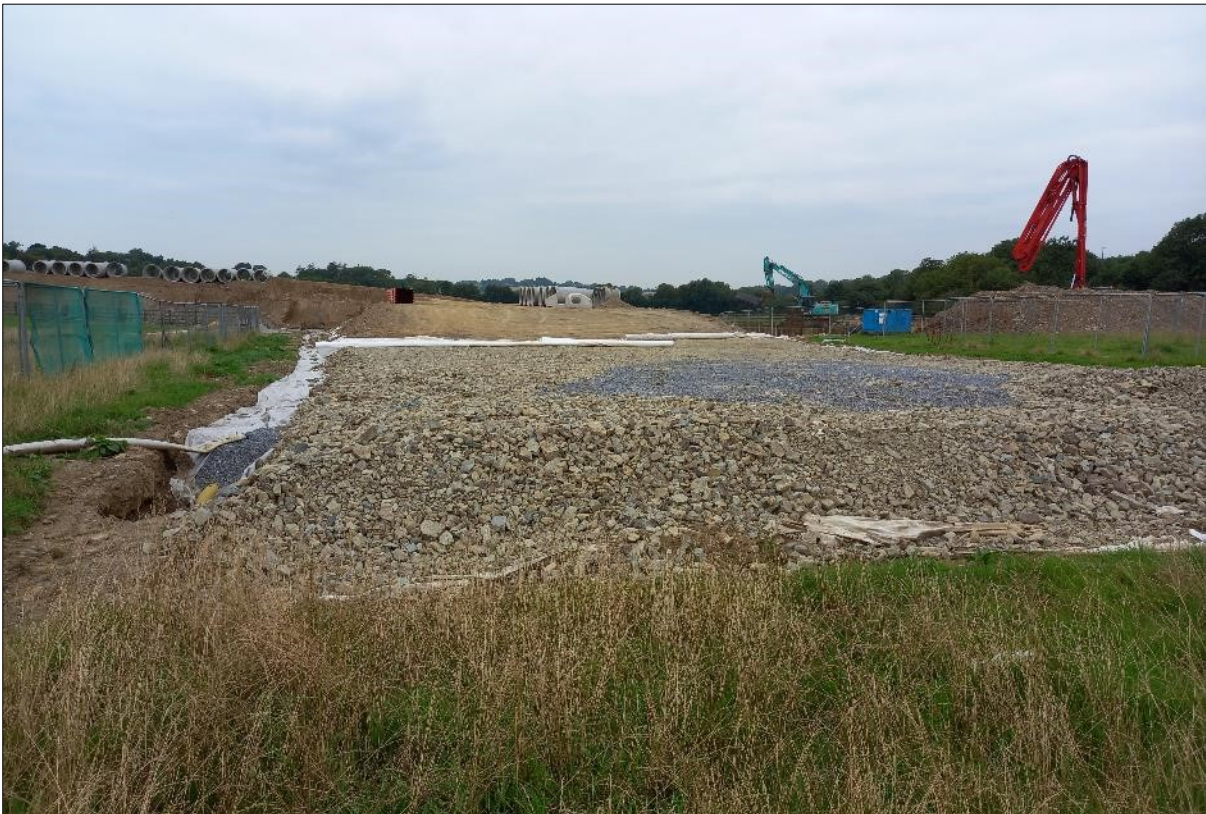
Plate 10: View of the hardstanding area constructed within the SHD boundary during the Relief Road works. This is the area of the feature noted on aerial imagery of the site
